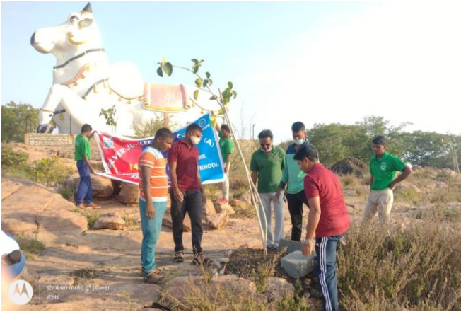
Lt. Sunil Kanna is helping and guiding the Cadets to install the Cement Bricks properly.
